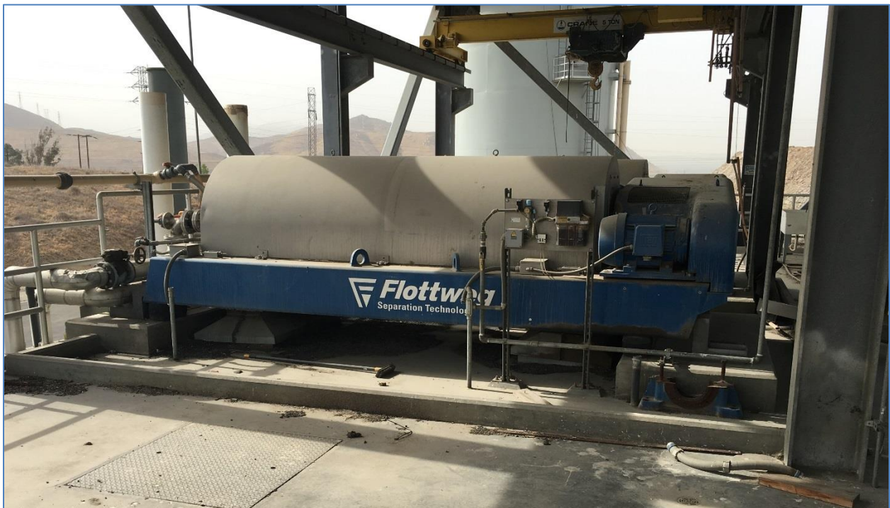
Figure 2-7 One of Two Existing Centrifuges
