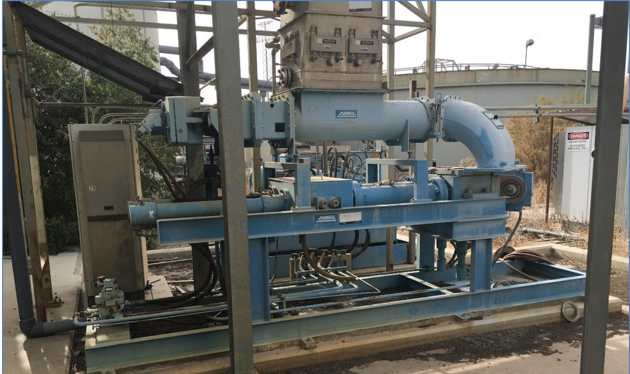
Figure 2-6 Existing High-Pressure Feed Pump
