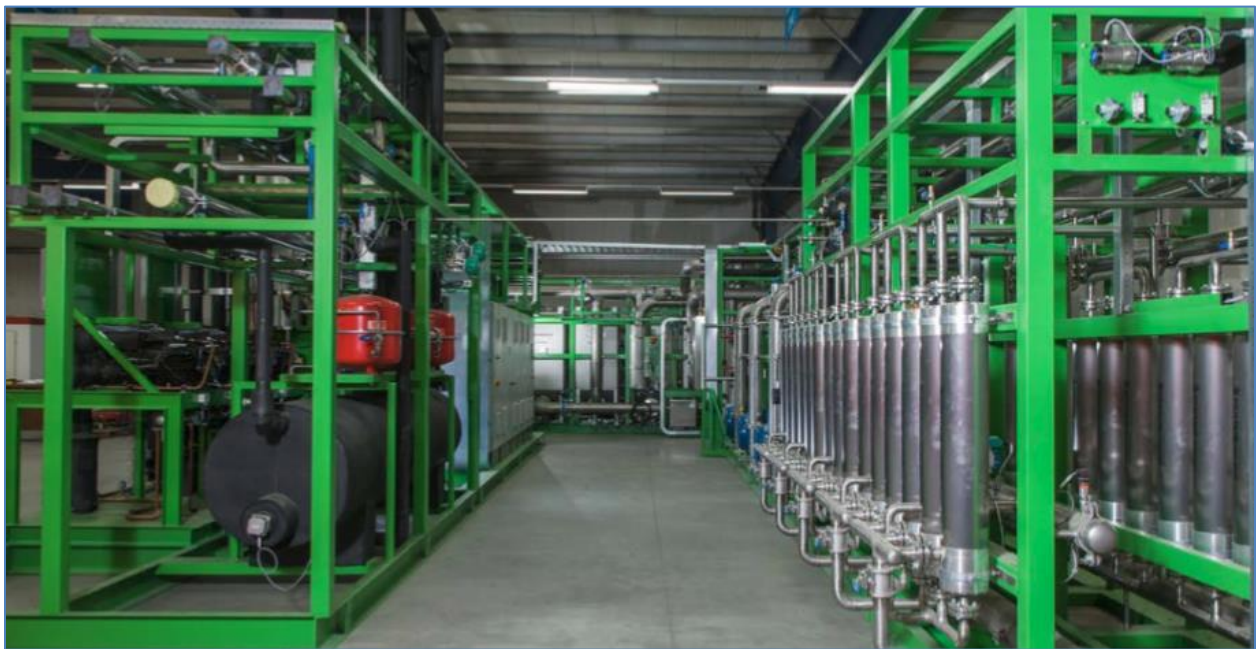
Figure 2-12 Biogas Upgrading System
