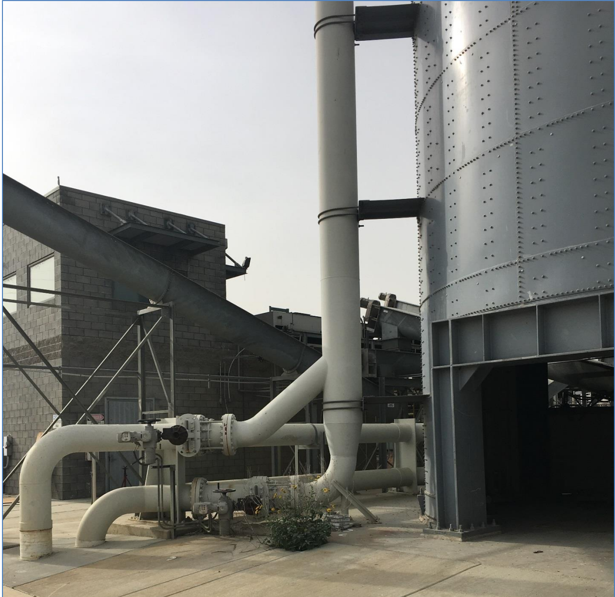
Figure 2-4 One of Two Existing Storage Silos with Supply Piping
