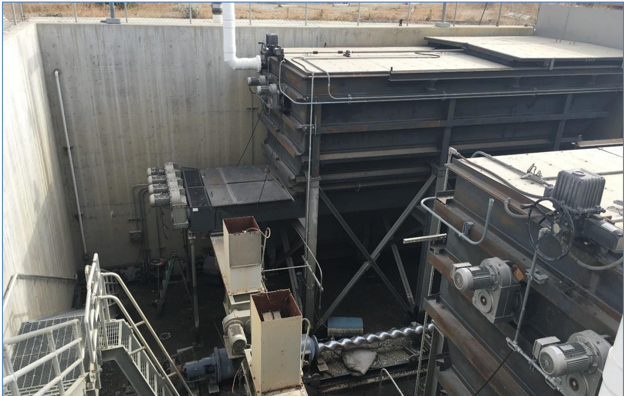
Figure 2-3 Existing Live-Bottom Receiving Bins
